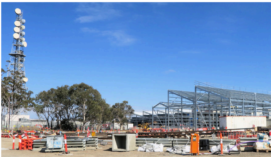
View from the north of construction underway at the new Maidstone Depot, 19 August 2024.
